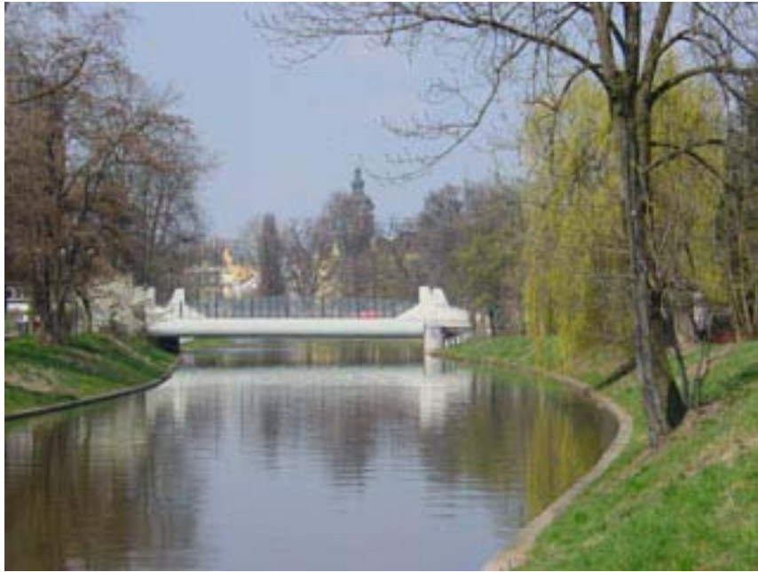
Fig. 1: The bridge over the River Malše in Mánesova Street causes water resources officers great anxiety, especially with swelling.
